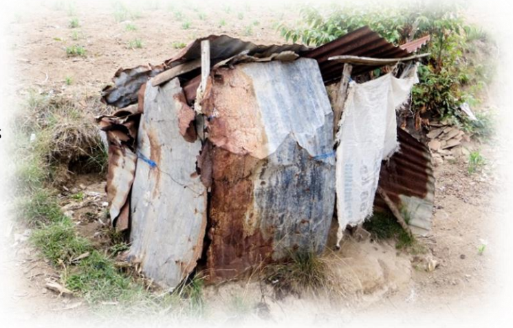
A typical toilet in rural Guatemala
